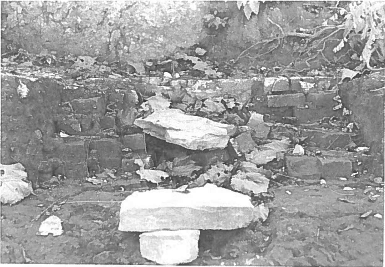
Figure 7. Photograph of the Fire Box Area of the Lower Rudd Lime Kiln on October 29, 1998 After Several Years of Erosion. Photograph is facing south.
