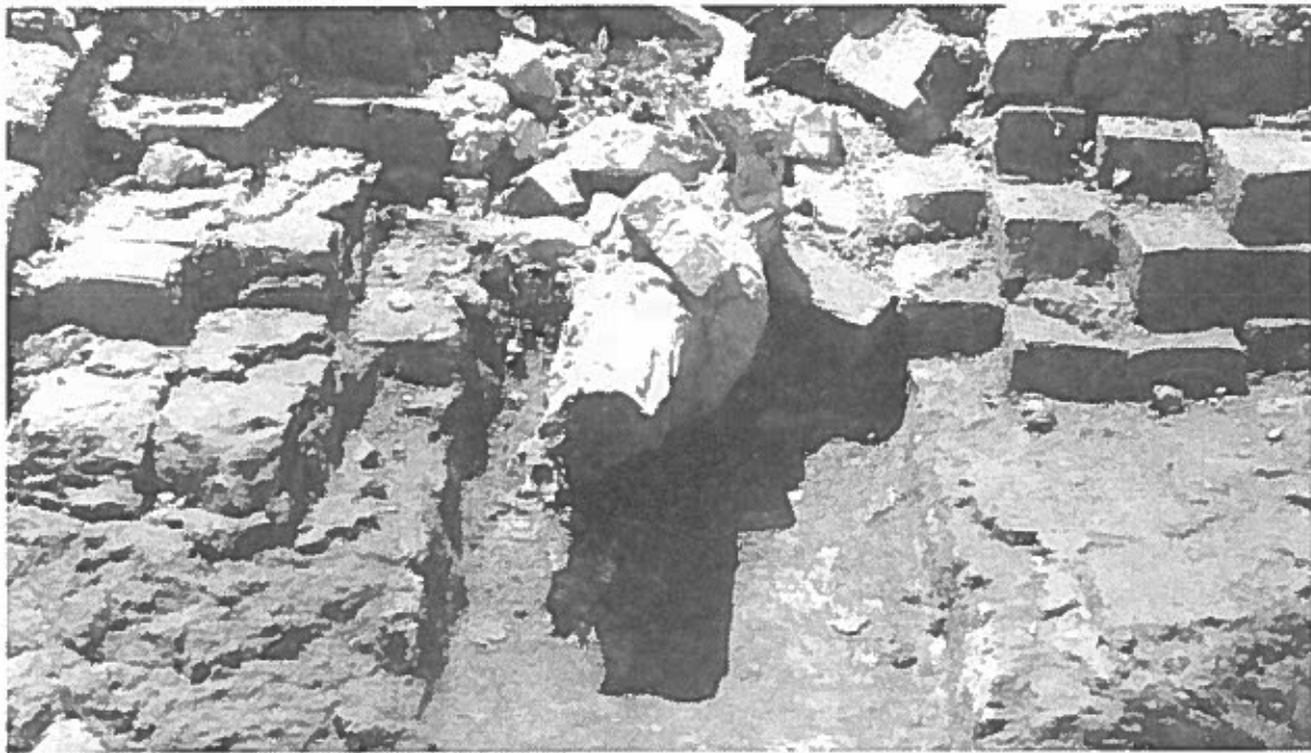
Figure 3. Photograph of the Fire Box or Drawing Area at the Base of the Lower Rudd Lime Kiln. The trough is in the bottom center with intact brick work on each side of a large tree root. The photograph is facing south.
