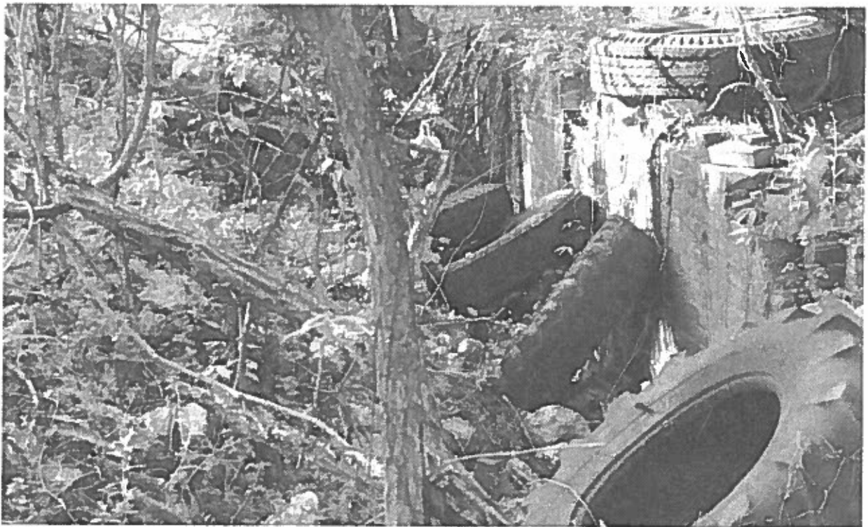
Figure 6. Photograph of a Surviving Brick Wall at the Northern End of the Incline (Area H). Photograph facing northwest.
