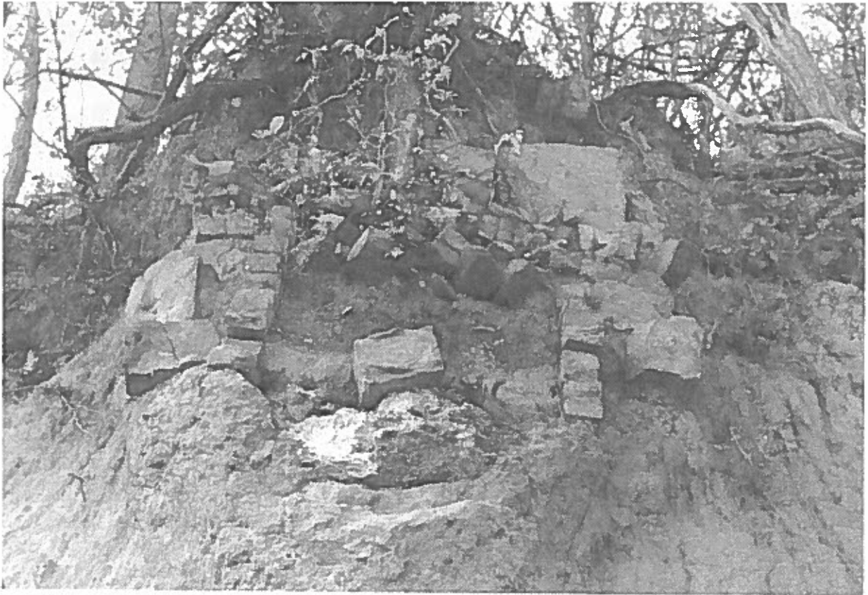
Figure 12. Close-up Photograph of the Upper Rudd Lime Kiln Showing the Fire Box and Remaining Lime (white area in lower center) Taken on October 29, 1998. Please note the base of the tree that grew into the kiln. The photograph is facing south.
