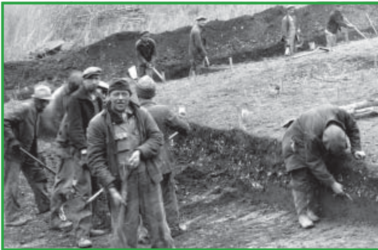
It's all in a day's work at this Muhlenberg County site: digging out the dirt and cleaning up the trench walls.
