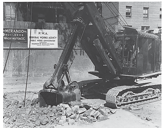
PWA Construction Site in Washington, D.C., 1933 (Franklin Delano Roosevelt Presidential Library & Museum. Digital Archive online. http://www.fdrlibrary.marist.edu/ , hereafter FDR Library)
