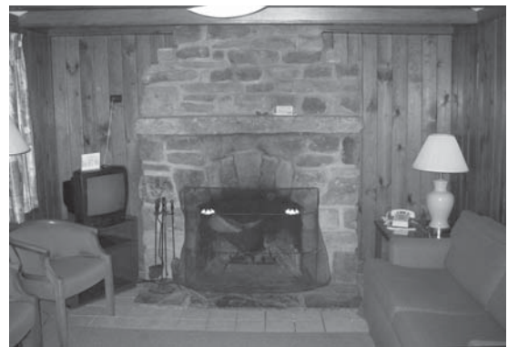
Fireplace at cabin 521. Note the altered wall surfaces and the original stone chimney. Photo taken in 2004.
