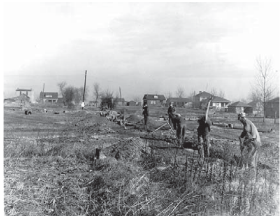
Workers at a City-Wide Sanitary Sewer project in Worthington (Greenup Co.). Photo date unknown. (GP Collection).
