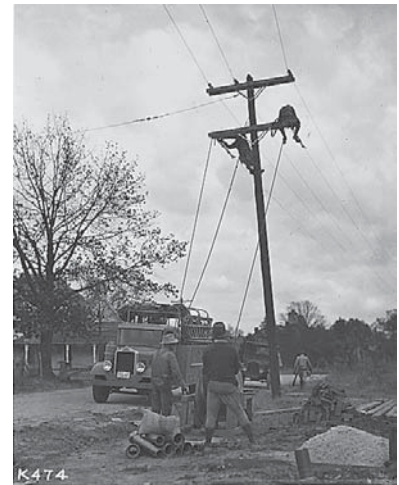
Stringing rural transmission lines in TVA service region. Date unknown. (FDR Library)
