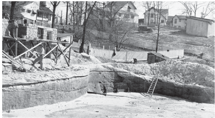
“Construction of a concrete swimming pool, 65’ x 100’, in the public park at Stearns, KY.” Photo taken 16 April, 1936. (GP Collection).
