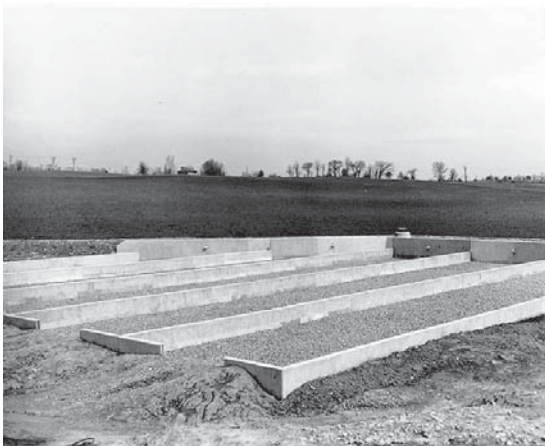
Slush drying beds at Danville (KY) sewage disposal plant. Photo date unknown. (GP Collection).
