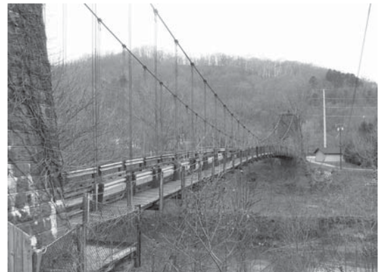
Pauley Bridge in Pikeville. A WPA project. Photo by Burgess and Niple, Inc. 2005.
