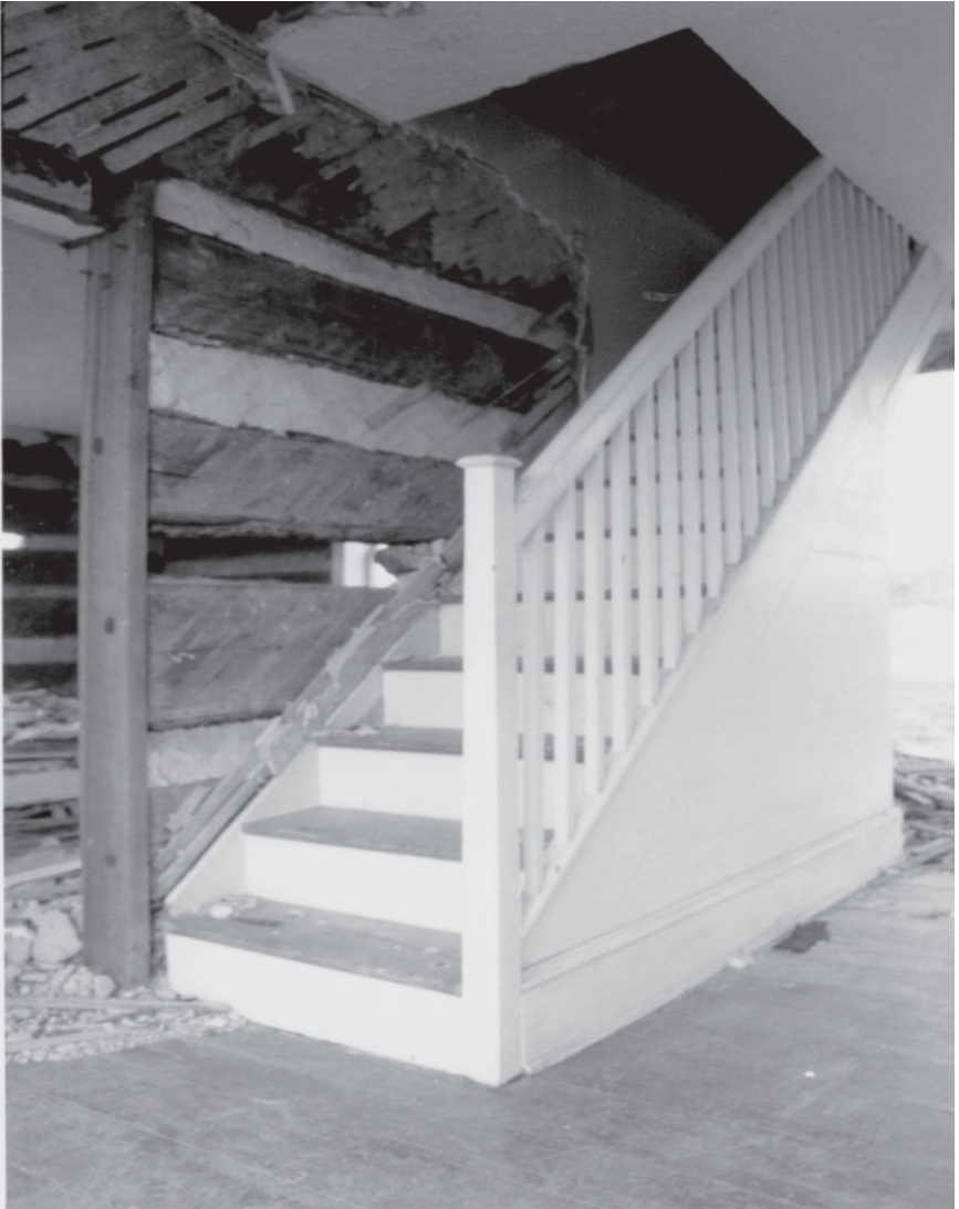
Staircase, Sullivan House, Franklin County, Circa 1810-1820. Note the chinking, plaster lath, and pegged door jamb. For another view of the Sullivan house, see figure 7.
