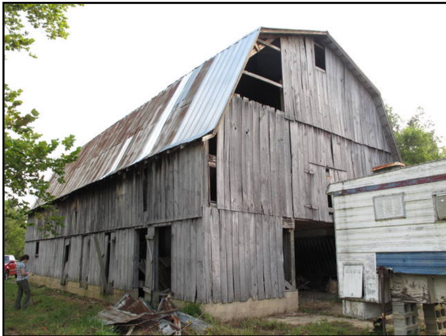
Figure 3. 47 Rear of the Rogers dairy barn (LV-76). A silo used to sit at the location of trailer (far right in photo).
