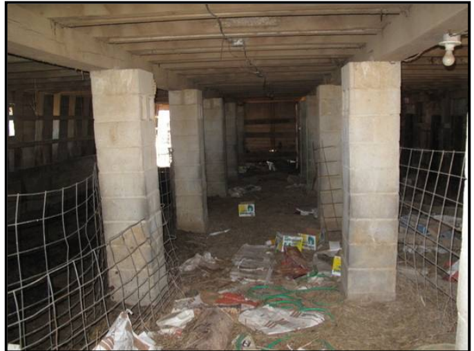
Figure 3. 30 Interior of the concrete block barn, CN-32, at the O.B. McDaniels Farm.
