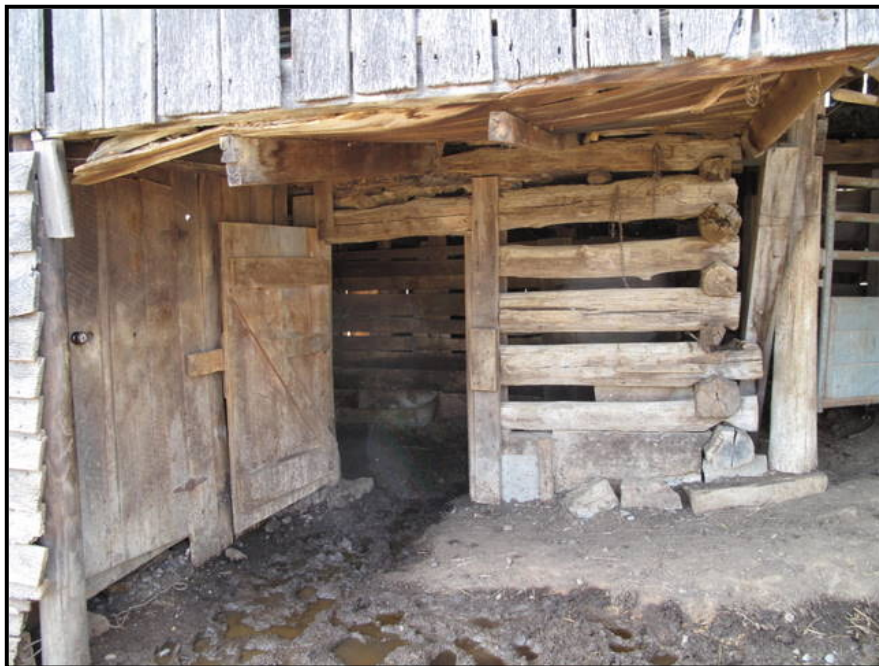
Figure 3. 21 Left hand side crib at CN-67.
