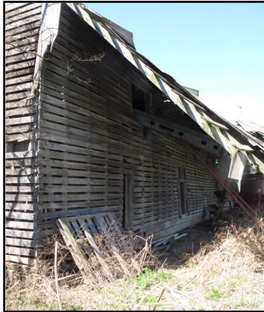
Figure 3. 68 North side of CN-32, showing cribs.
