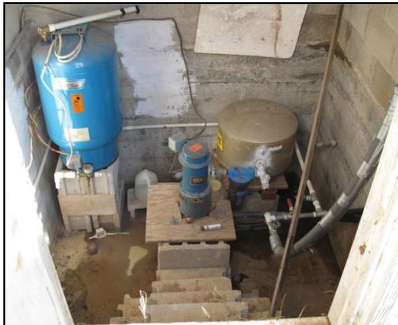
Figure 4. 37 Interior of pump house at CN-71.
