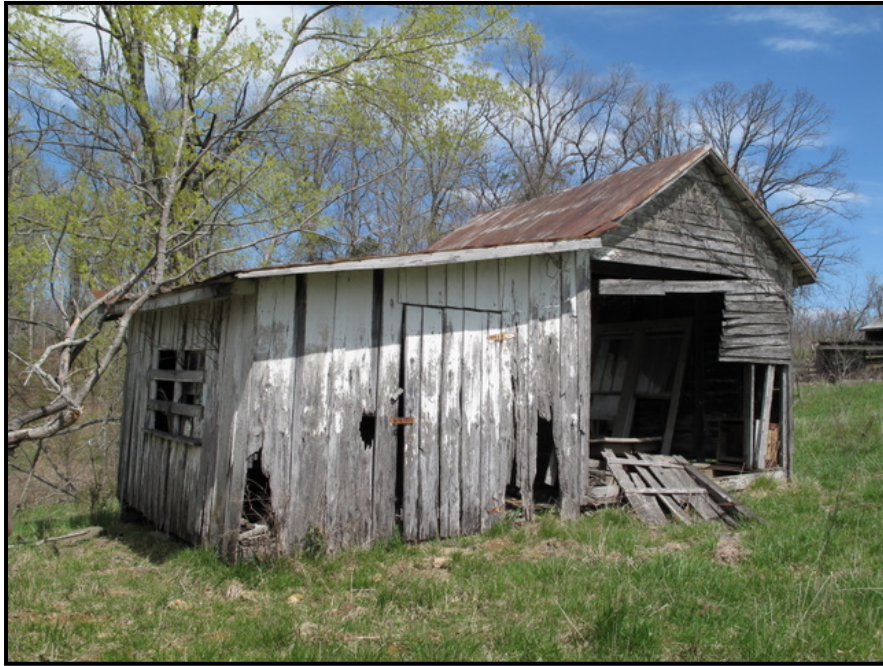
Figure 4. 10 Dilapidated meathouse with side shed addition at LV-54.
