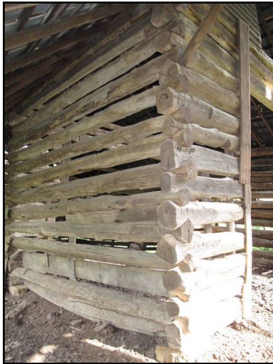
Figure 3. 18 Detail of notching on CN-26.
