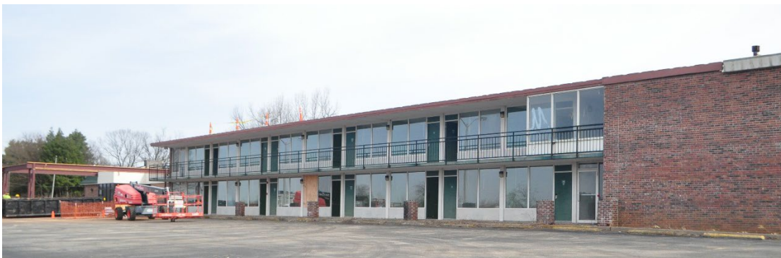
Figure 08: Original flat roof is once again exposed after removal of non-historic materials, Feb. 2023
