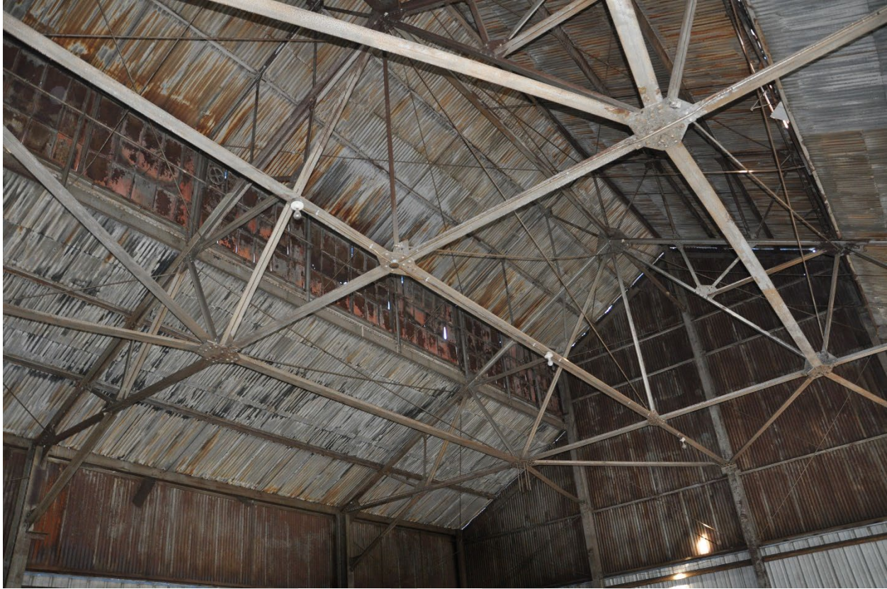
Figure 17: Detail of the Fox Fink steel truss system supporting the roof of the main block of the Magnus Metal Company Building.
