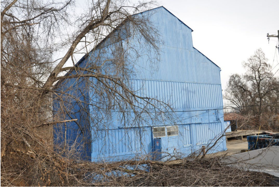
Figure 5: Façade (southwest) and northwest elevations of the main block of the Magnus Metal Company Building, looking southeast.
