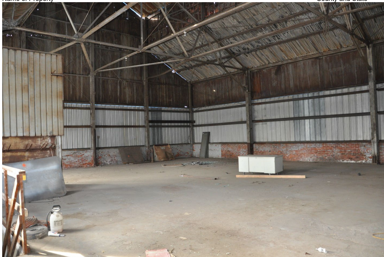
Figure 15: Interior view of the second story of the main block of the Magnus Metal Company Building, looking southwest.
