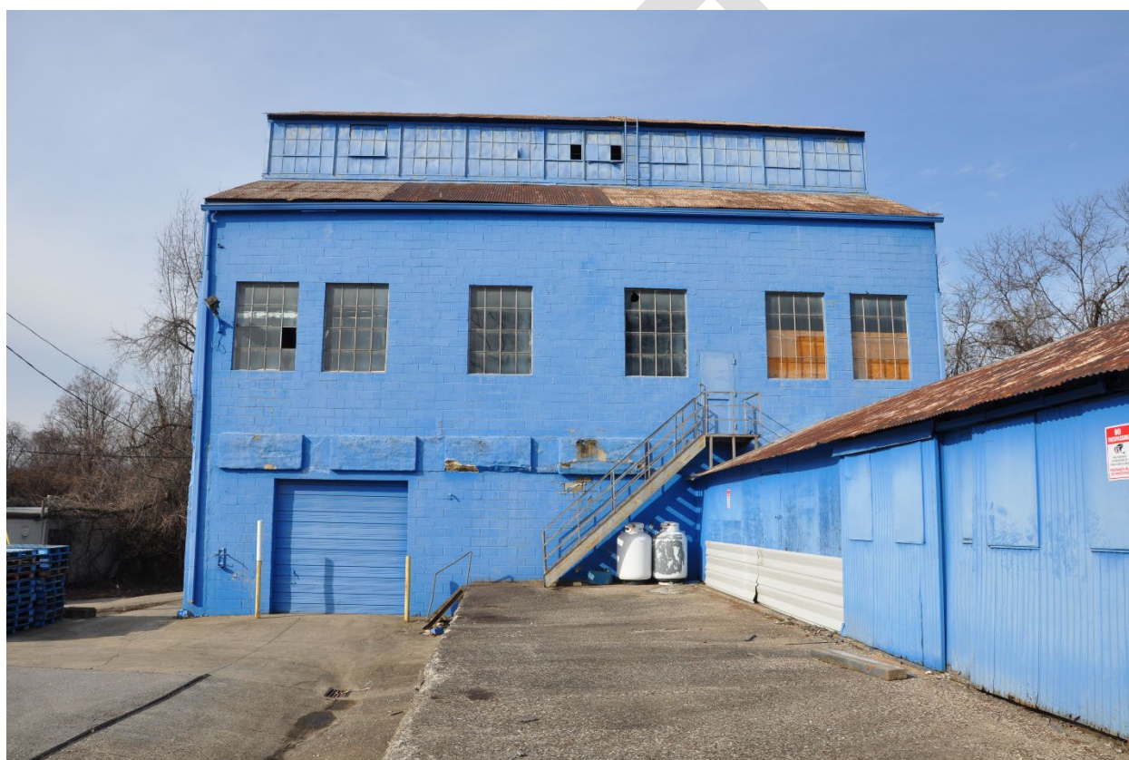
Figure 7: Southeast elevation of the main block of the Magnus Metal Company Building, and partial view of the southwest elevation of the addition, looking west-northwest.
