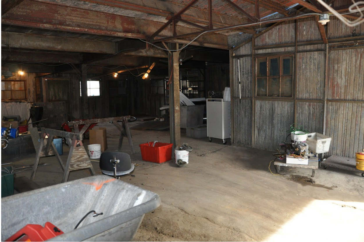
Figure 18: Interior view of the first story of the first and second additions of the Magnus Metal Company Building, looking northeast.
