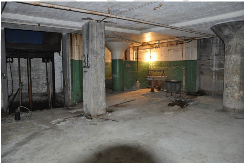
Figure 21: Interior view of the basement of the main block of the Magnus Metal Company Building, including the elevator shaft and the sink, looking southeast.
