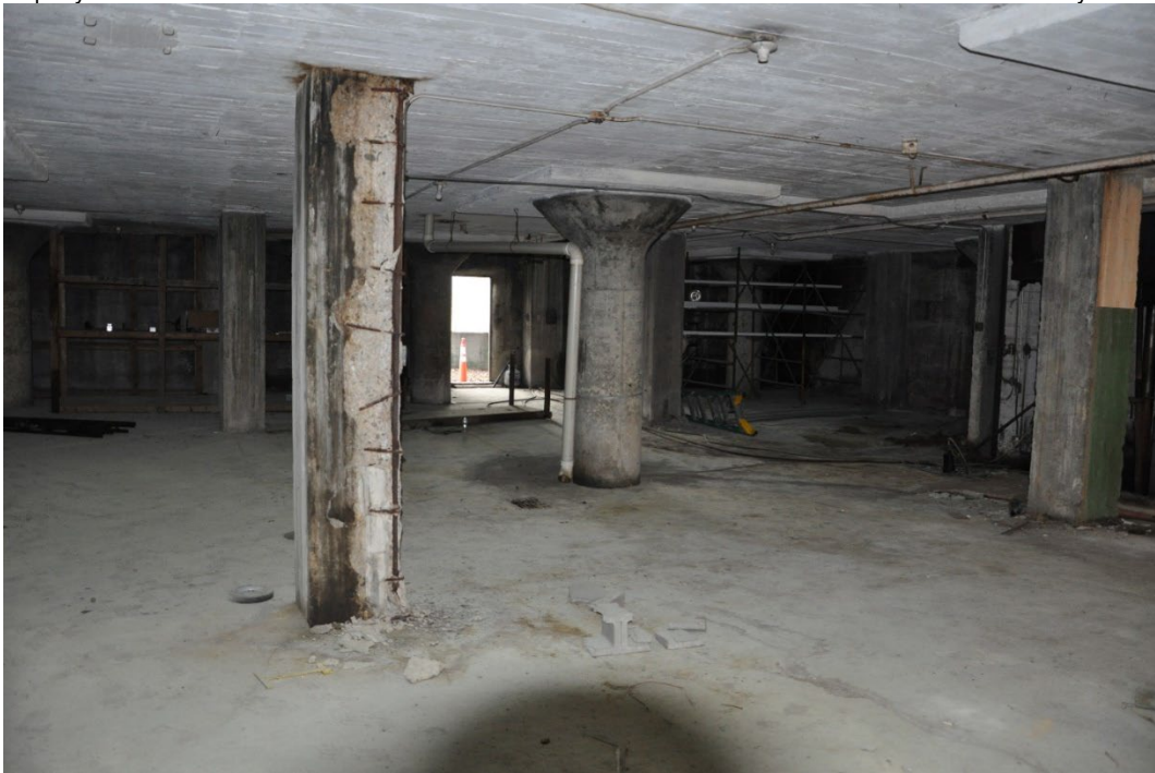
Figure 20: Interior view of the basement of the main block of the Magnus Metal Company Building, looking northeast.
