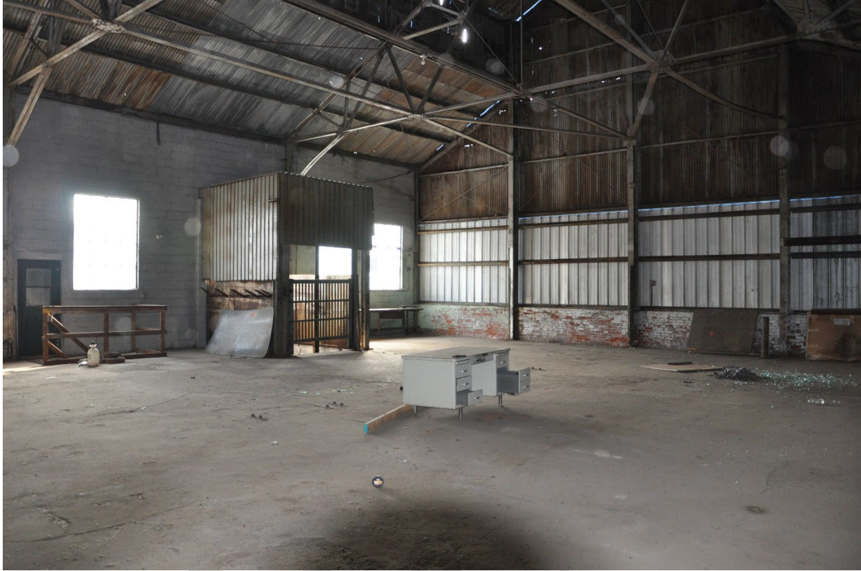
Figure 16: Interior view of the second story of the main block of the Magnus Metal Company Building, including the elevator shaft, looking southeast.
