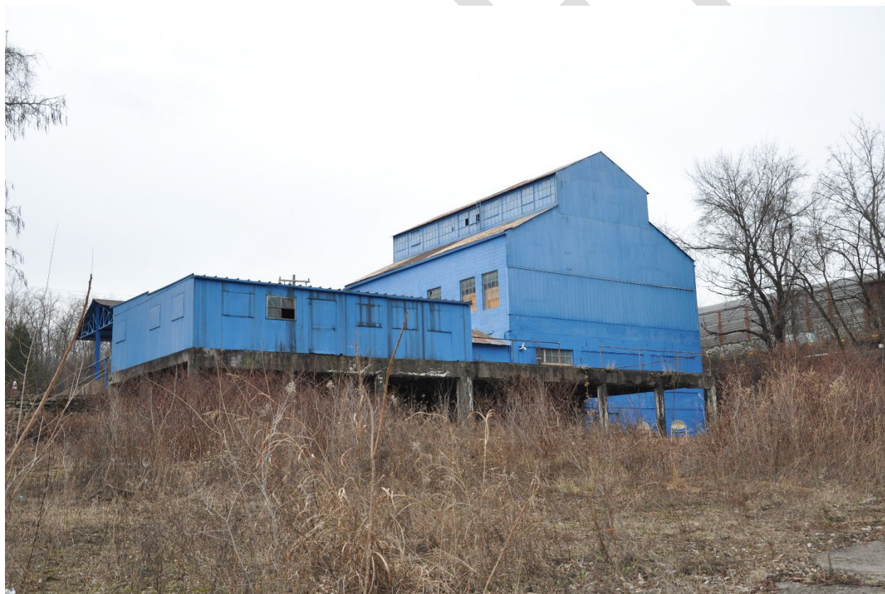
Figure 8: Southeast and northeast (rear) elevations of the addition of the Magnus Metal Company Building, and northeast (rear) elevation of the main block, looking southwest.
