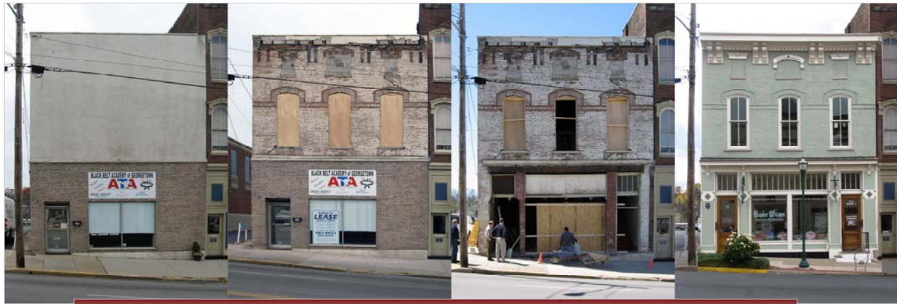
Pullen Building, Georgetown, rehabilitated using state and federal historic rehabilitation tax credits
