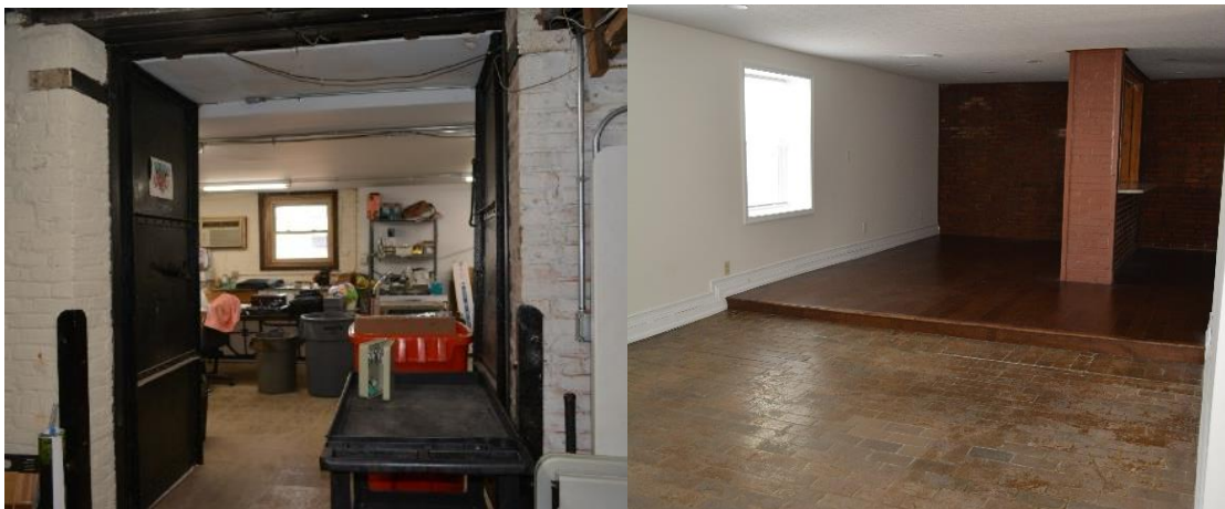
Iron fire door in storage area at rear of office; Brick floor in third floor apartment
