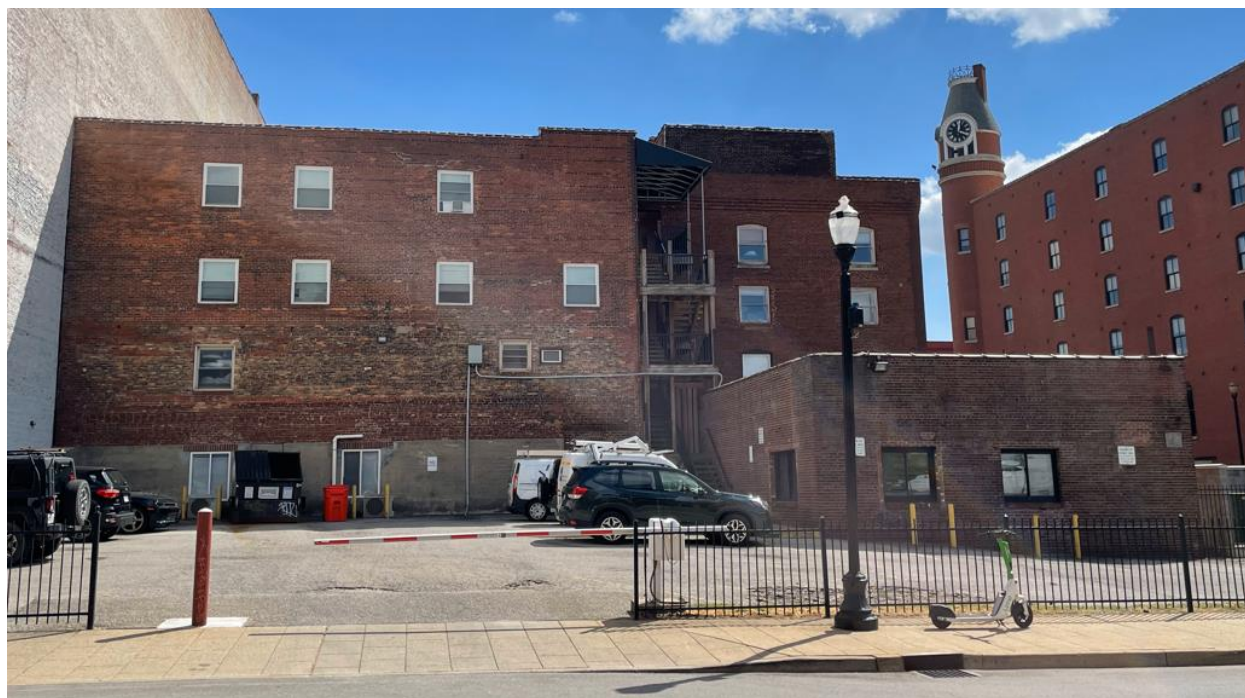
North/rear façade: eastern and western sections divided by hallway/stairway. Utility building at right.
