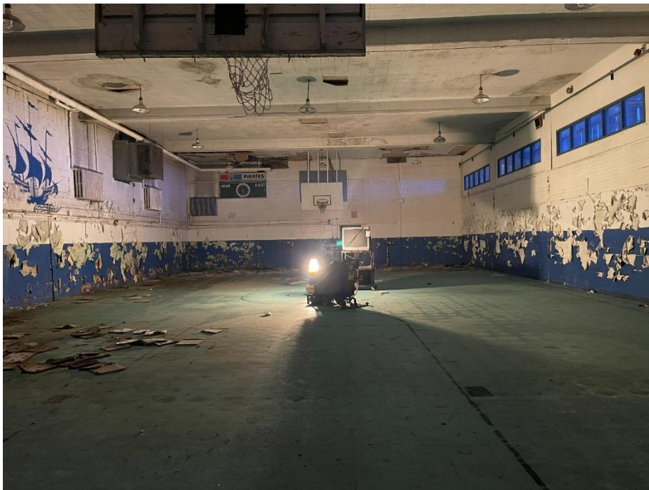
Gymnasium: Ship painting and large fan are located in 2 of the 5 original windows that have been filled with masonry. Windows in upper right overlook gymnasium from lower level. These windows were installed into large openings that allowed a view to gymnasium.
