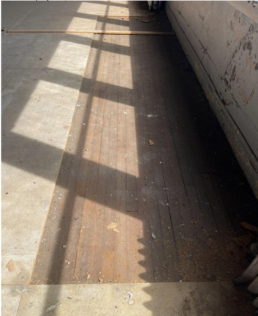
View of original hardwood floor after particle board was removed in third floor classroom.
