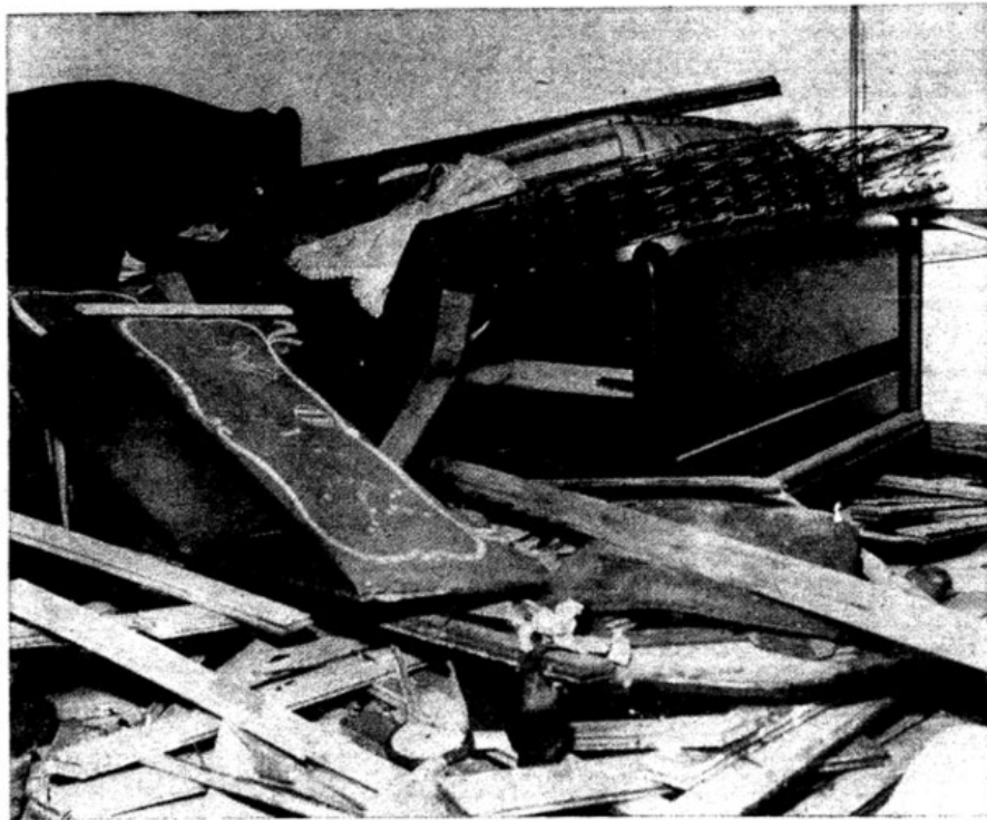
TOP PHOTO illustrates damage to the Wade home after a bomb had been planted. Notice impact of bomb separated the gray stone from siding. Bomb was planted beneath the Wade's bathroom. BOTTOM PHOTO shows how explosion uprooted floor boards and demolished furnishings in bedroom. No one was present in either of the rooms when bomb was detonated.
