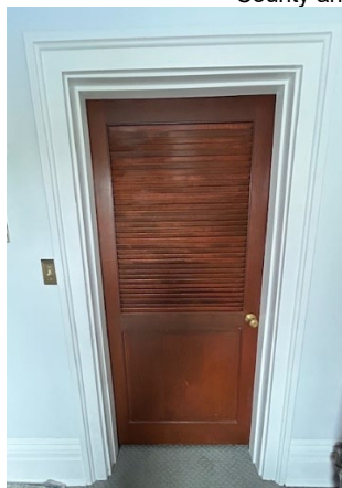
Door Trim of doorway leading to Master bedroom on wall opposite window
