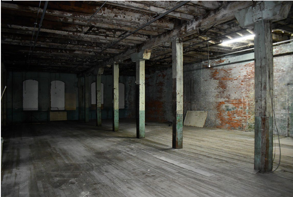
Figure 22 Second floor, open space characterized by the three rows of wooden posts and wooden floors. (0016)
