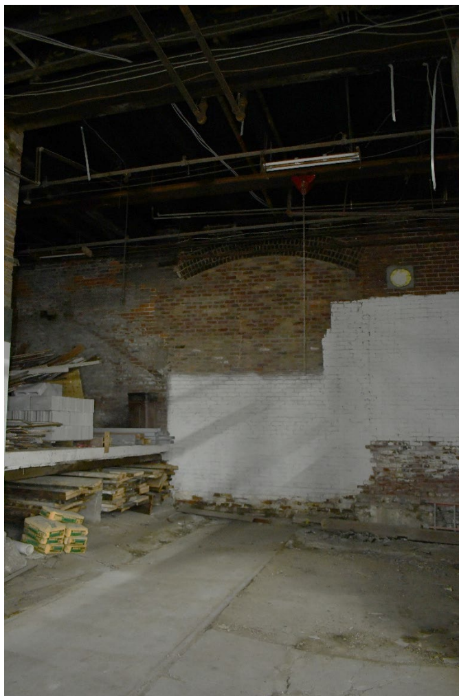
Figure 15 First Floor, railroad siding entrance (infilled with brick) on east elevation of building, note tracks infilled with concrete. (0009)
