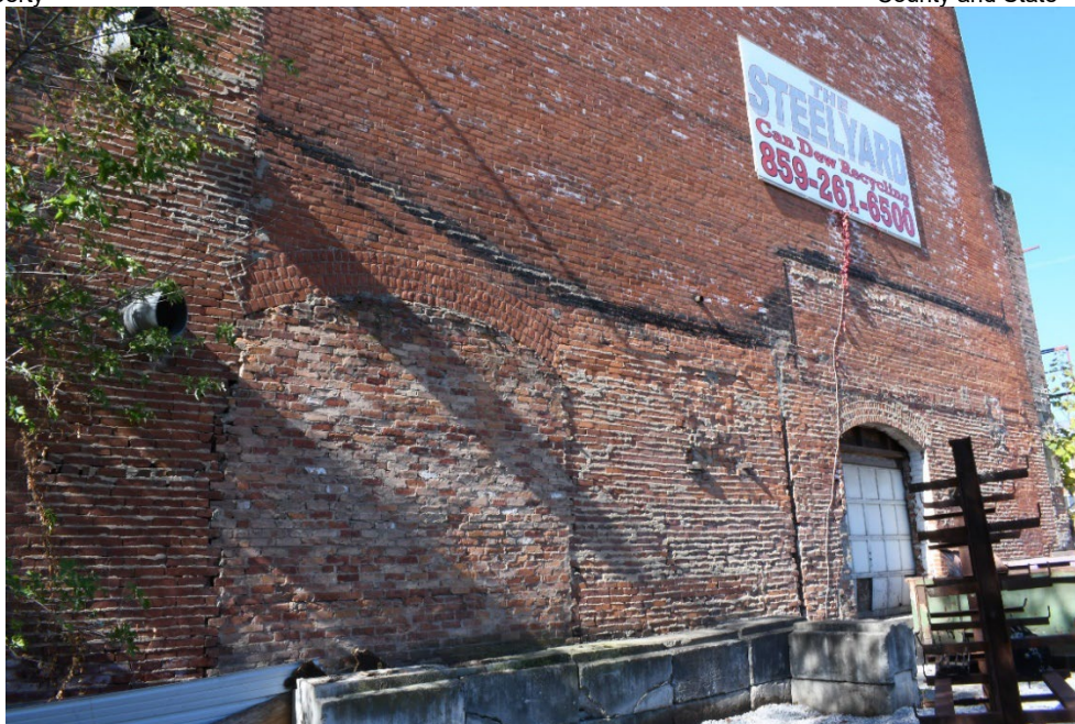
Figure 14 East elevation of Overman Schrader Cordage Company Building, looking NW, note brick filled bay and roofline ghosts from previous appendages. (0008)
