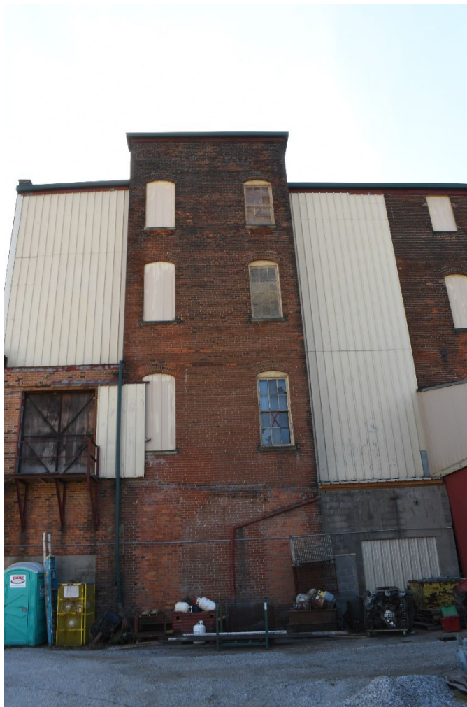
Figure 12 North elevation of Overman Schrader Cordage Company Building, looking south, tower, metal panels west and east, concrete block addition and brick addition. (0006)
