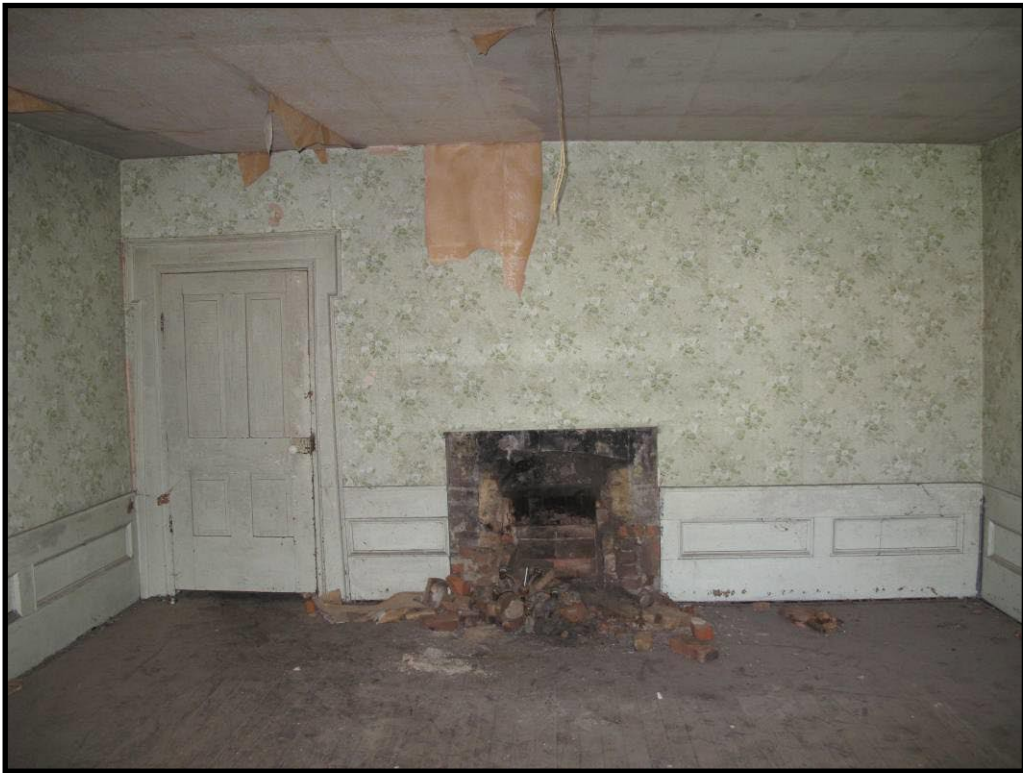
Figure 134 Interior of CS-85.
