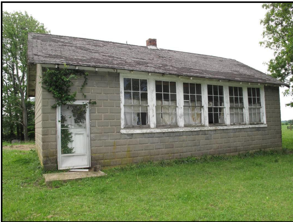
Figure 25 Duncan School, CS-99, a one-room concrete block school in the Eubank quad.
