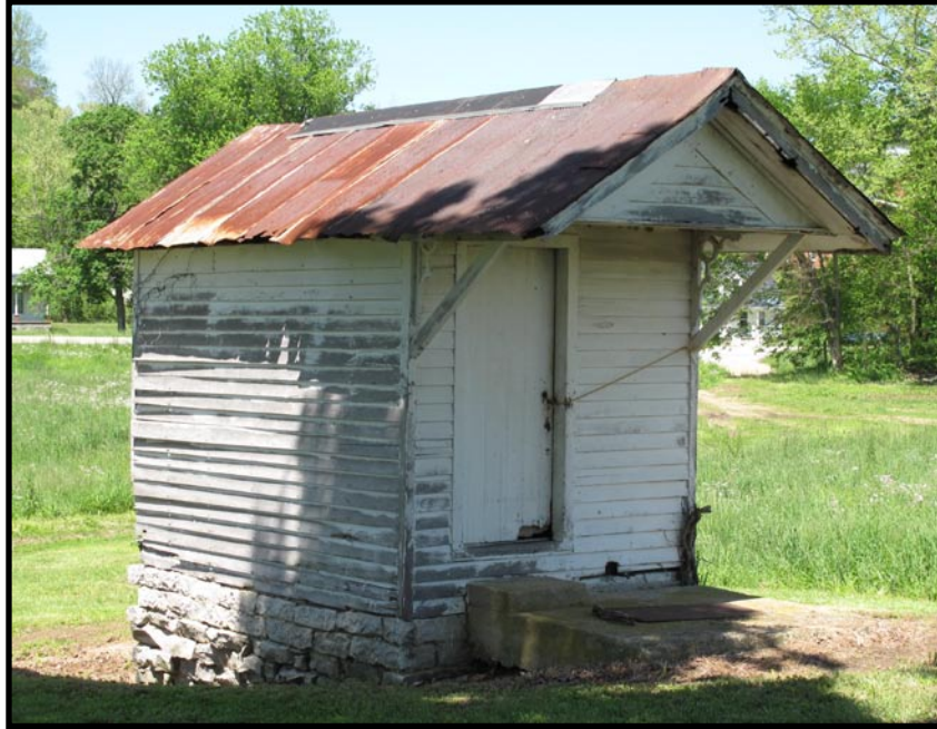
Figure 143 Springhouse and dry storage at the Pryor Prewitt House, CS-10, Ellisburg quad. Cistern access is in front, to right of door.
