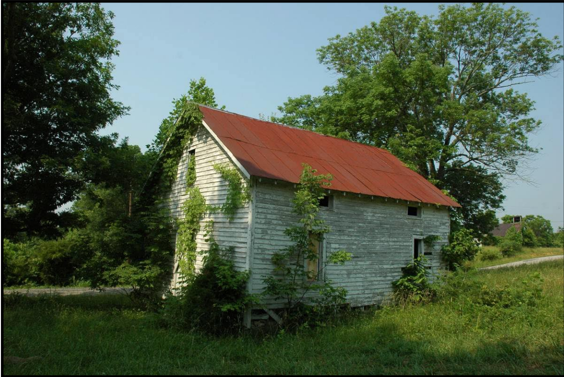
Figure 26 Patsy Riffe Ridge Schoolhouse, CS-126, a one-room school in the Hustonville quad.
