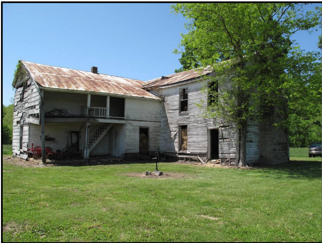
Figure 89 The rear and ell addition of the log and frame Pryor Prewitt House, CS-10.
