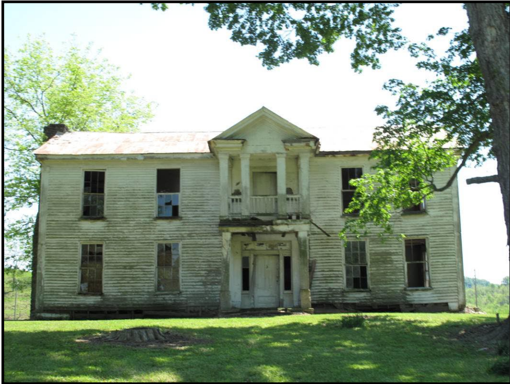
Figure 88 Façade of the log and frame Pryor Prewitt House, CS-10, Route 78 in Ellisburg quad.
