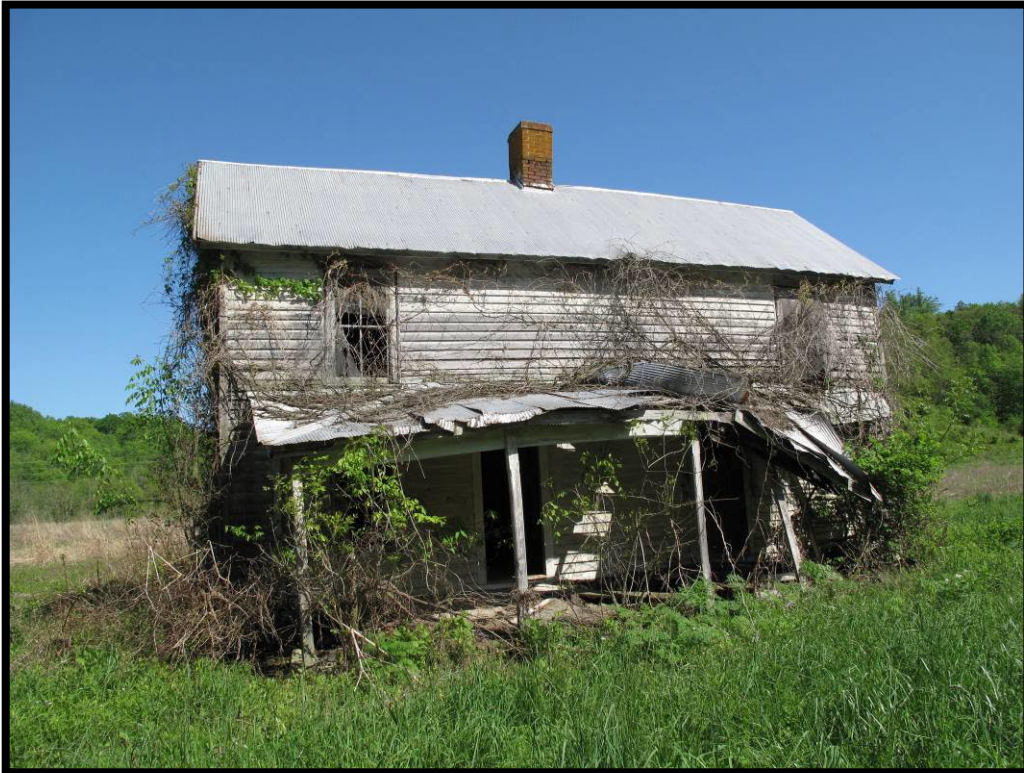
Figure 107 CS-91, an abandoned Cumberland on Long Hollow Road, Ellisburg quad.
