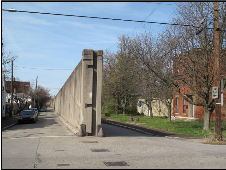
Figure 3. 38 A portion of the floodwall in Butchertown at Adams and Quincy Streets.
