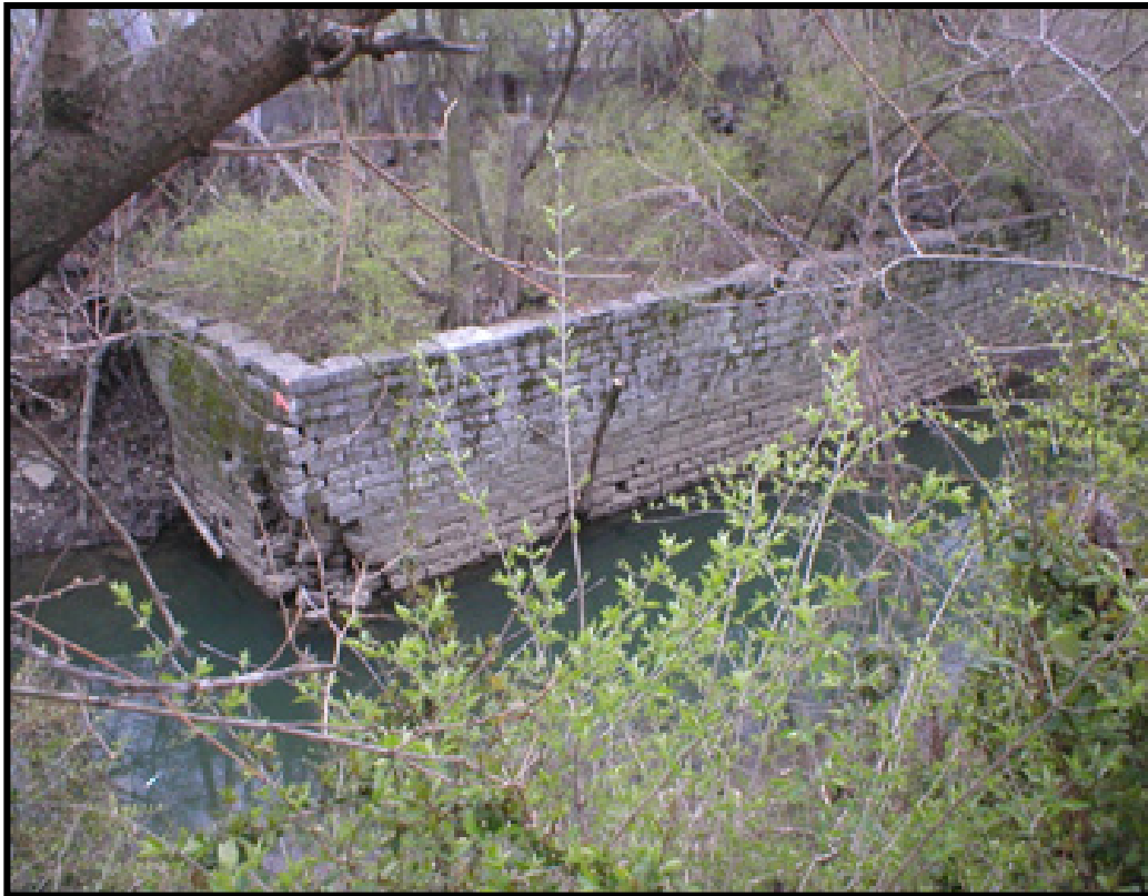
Figure 6.6 A stone foundation associated with a distillery at the Former River Metals industrial property along Beargrass Creek adjacent to Area 2.
