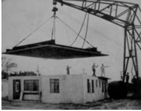
Putting the final prefabricated element on the concrete house manufactured by the Ibec Corporation. This prefab company used precast concrete panels for its houses. (Source: A Practical Guide to Prefabricated Houses ).
