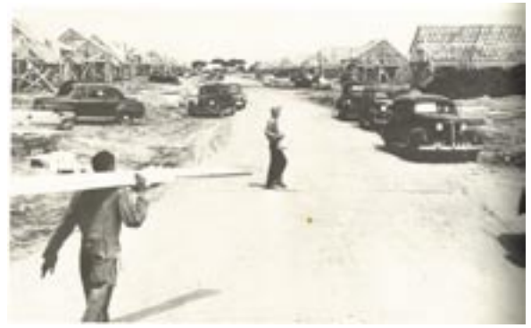
Tract housing being constructed at Levittown. (Source: Building Suburbia: Green Fields and Urban Growth, 1820 - 2000 ).
