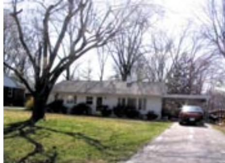
This Gunnison at 505 Minerva Place (MCNP-951) has had its original windows replaced with non-historic windows.
