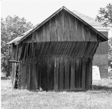
End View of the Humphrey-Milton Chicken House. The roosting area is slatted to allow waste to fall through to the outside of the building, where it could be easily collected for manure.
