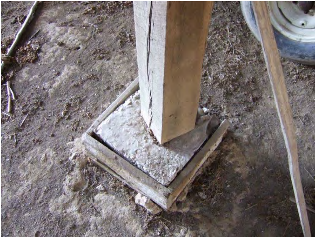
Figure 249: MN 602, Multi-purpose Transverse Frame Barn, late twentieth century, Bradfordsville vicinity: detail of post on cement foundation block. See also Figure 251.
