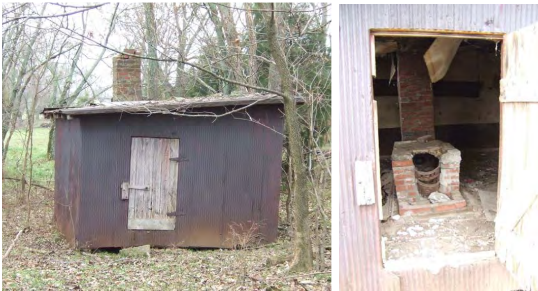
Figure 299: WS 436, Joe Rine's Brooding house, 1930s-1940s, Springfield vicinity: exterior, left, and interior, right, showing warming stove.
