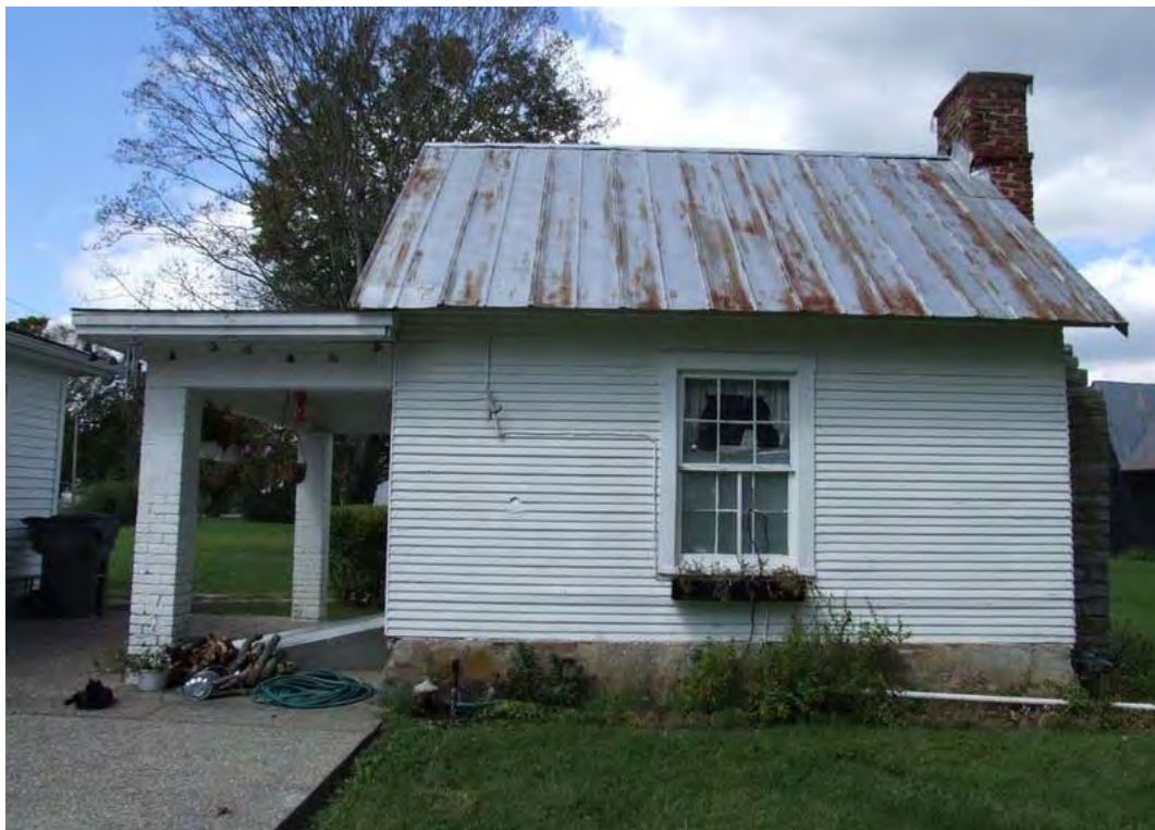
Figure 211: WS 33, Kitchen, mid nineteenth century, Maud. The porch is an early twentieth century addition. The building later served as the Maud Post Office.
