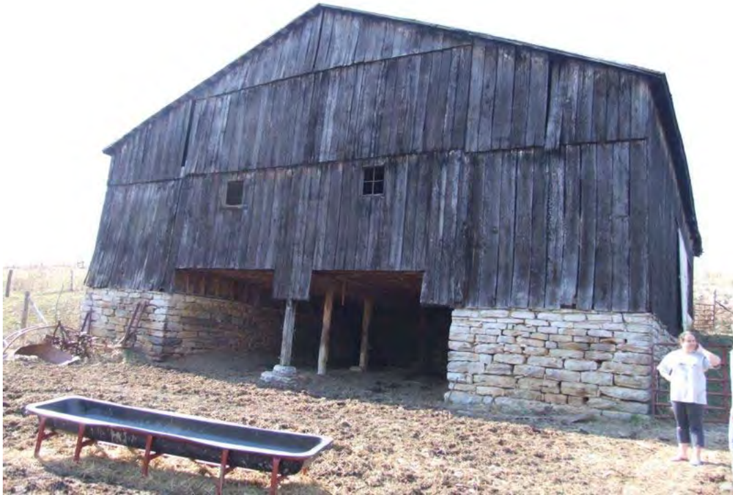
Figure 241: WS 633, Stock Barn, mid-late nineteenth century, Deep Creek vicinity. See also Figure 242.
