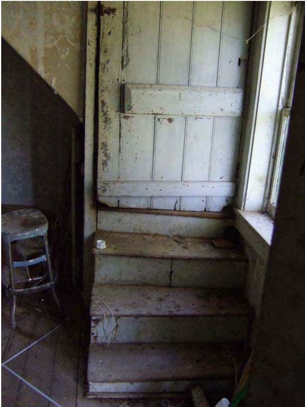
Figure 32: WS 316, Slack's Cabin, mid-late nineteenth century, near Fredericktown: interior detail showing corner stair and door. The door is a historic example of architectural material that has been salvaged and reused. See Figure 129 for exterior view.
