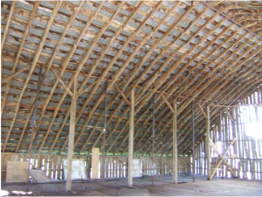
Figure 252: WS 314, Dairy Barn, early twentieth century, interior view of loft, Fredericktown vicinity. See also Figure 277.
