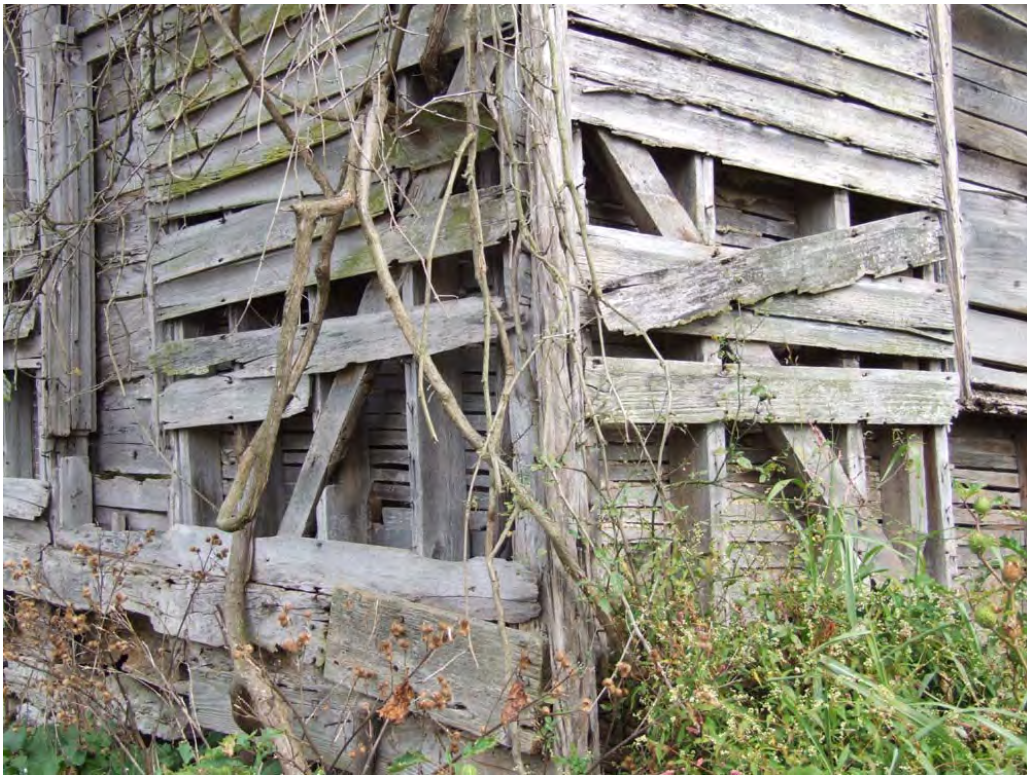
Figure 15: WS 359, Frame House, 1860s-1880s, Maud vicinity. Detail of nailed frame with corner braces.
