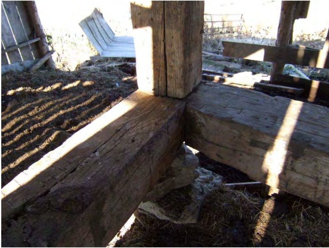
Figure 248: WS 451, Timber Frame Barn, nineteenth century, Polin vicinity, detail of sills and post. See also Figure 250.
