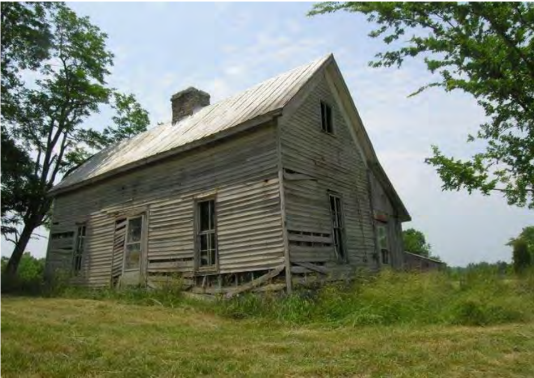
Figure 5: WS 972, Cooksey House, central chimney double pen, mid-late nineteenth century, Willisburg vicinity. The resource itself is a document of the past.
