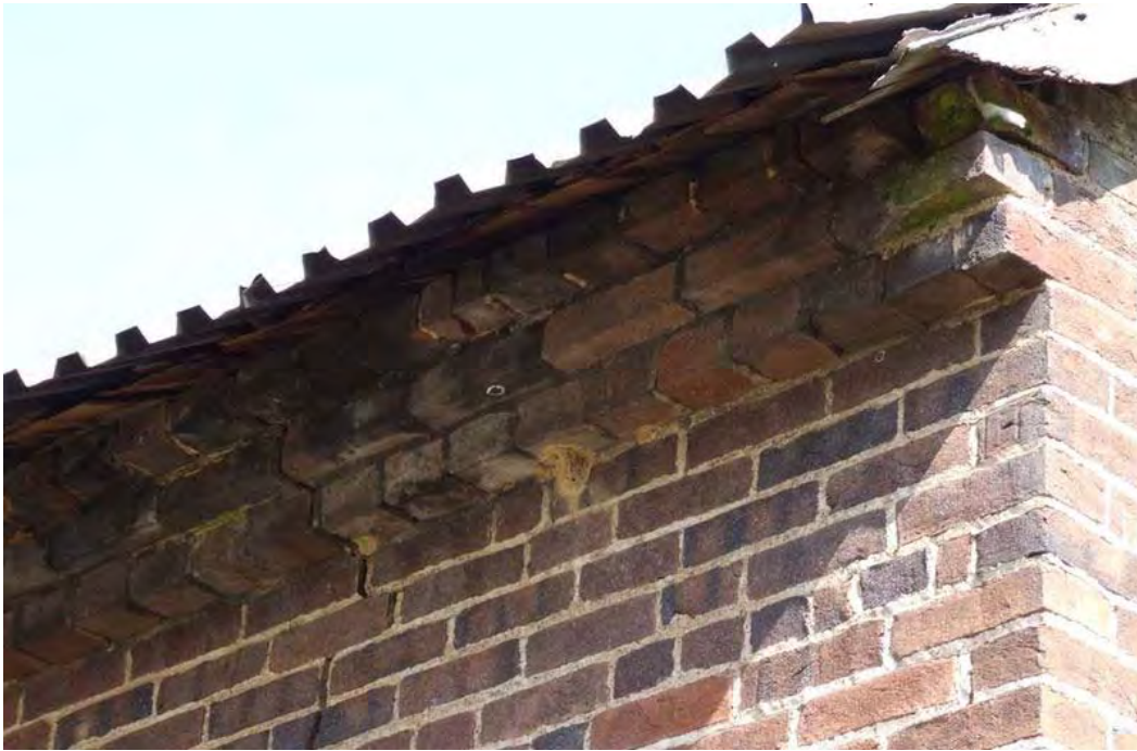
Figure 19: WS 15, Meathouse, early 19 th century, 1840s, Fredericksburg vicinity. A good example of a corbelled eave.
