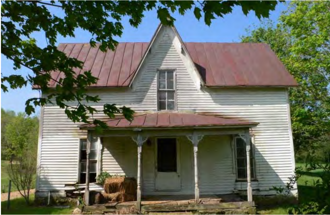
Figure 45: MN 683, Balloon frame single cross gable Gothic/eclectic style house, 1860s-1870s, Bradfordsville/Gravel Switch vicinity. See also Figure 43, Figure 46, and Figure 47.
