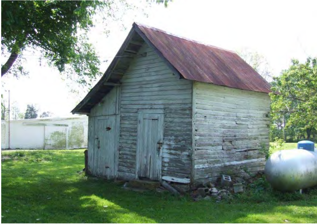
Figure 210: MN 567, Meat- or Smokehouse, New Market, late nineteenth-early twentieth century. Meat houses frequently have side shed appendages used for various functions such as tool storage.
