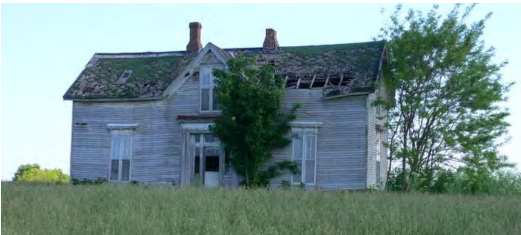
Figure 53: MN 688, Glasscock house, mid nineteenth century, Beech Grove vicinity. See also Figure 54, Figure 77, and Figure 80.
