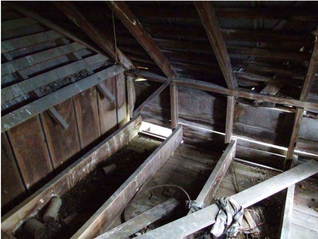
Figure 73: WS 247, Detail of attic framing in wing where it joins the main body of the house. The original house is vertical plank frame, the addition is light balloon frame. See also Figure 72.
