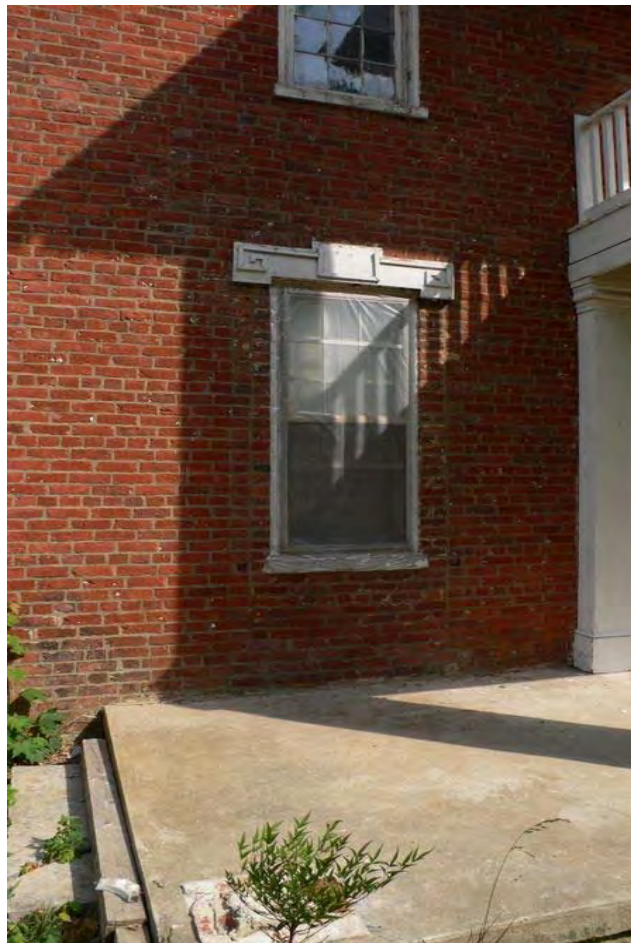
Figure 29: MN 919: detail of window to left of front door with brick infill scar indicating the opening was once a doorway.
