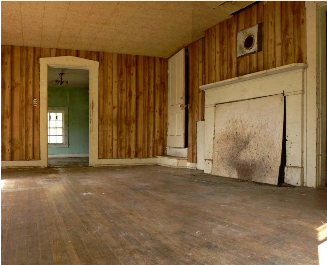
Figure 46: MN 683, Interior of left hand room, showing Greek style mantle & door surround. See also Figure 43, Figure 45, and Figure 47.
