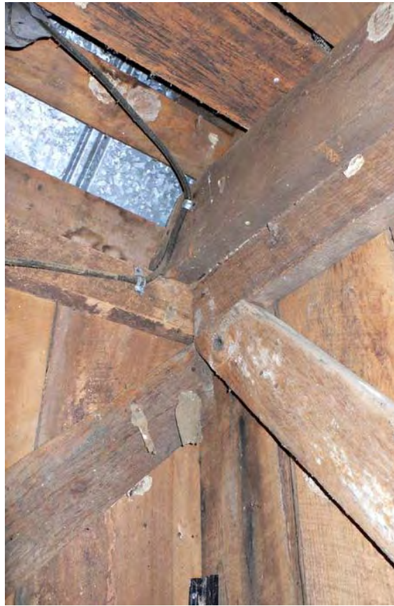
Figure 17: MN 685, Frame House, late nineteenth century Gravel Switch vicinity. Detail of interior corner bracing in a vertical plank frame building.
