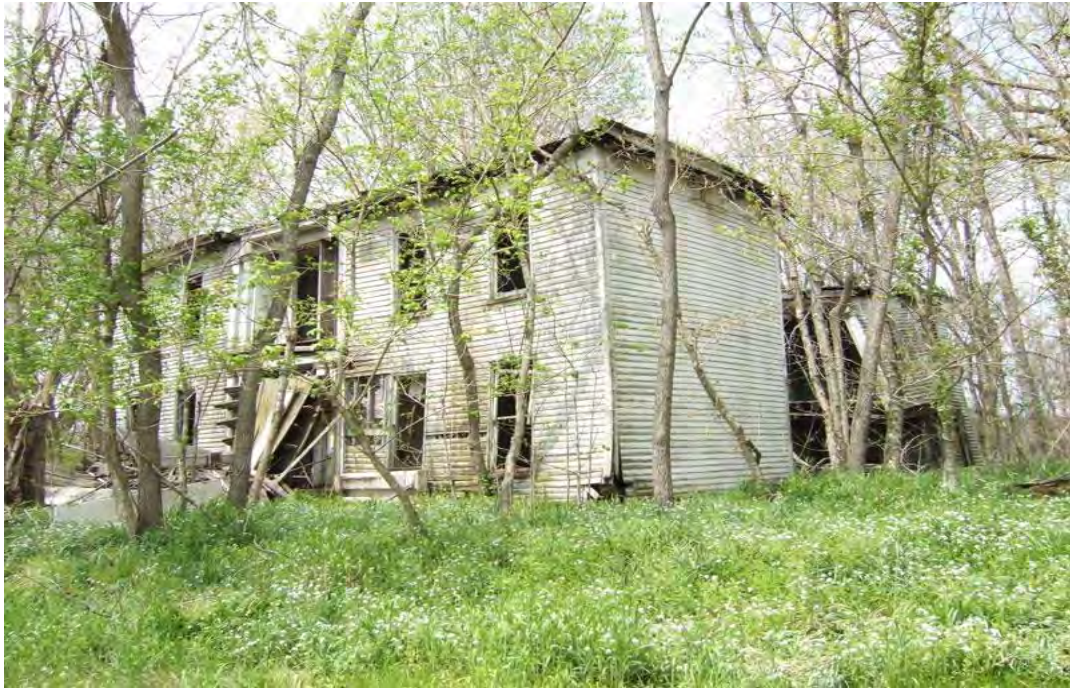
Figure 39: MN 1, Bradford Place, second quarter nineteenth century, Bradfordsville Vicinity. Now badly deteriorated, the Bradford house has elements of Greek Revival and Italianate styles. See also Figure 40.
