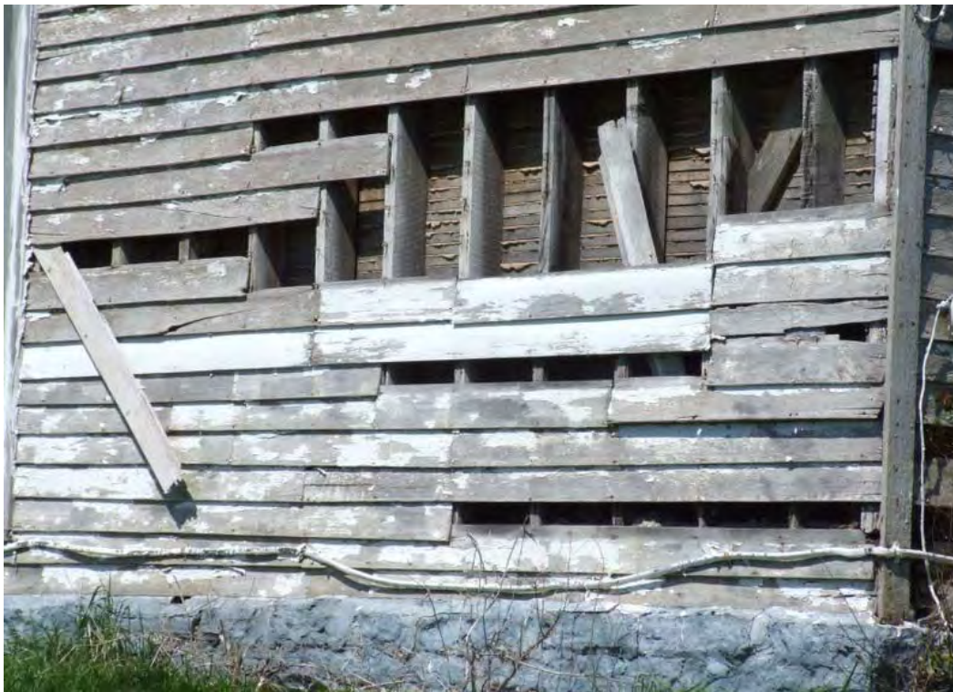
Figure 16: WS 721, Frame House, 1870s-80s, Cisselville vicinity. Detail of stud balloon framing, in this case with 2 x 6 studs rather than the 2 x 4 that ultimately became the standard.
