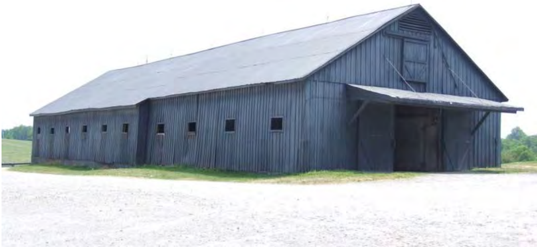
Figure 268: WS 878, Horse Barn, early-mid twentieth century (built in two stages), Kalarama Saddle bred Farm, Springfield.
