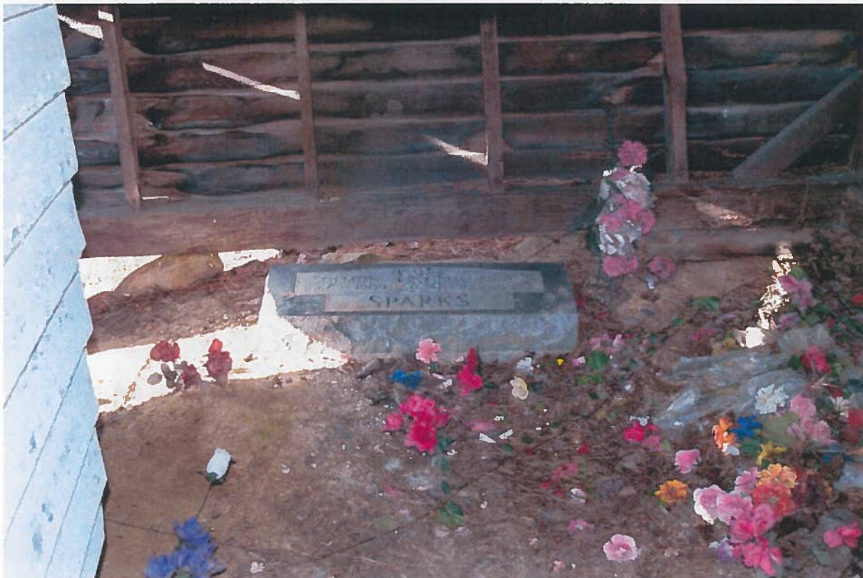
Caption: "Little" Sparks Grave House Interior Showing Framing of Building and Headstone Inside
